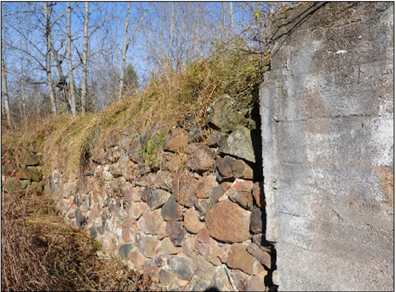
Interior view of north section of wall, detailing two different construction methods. Photo by M. Schweitzer.
