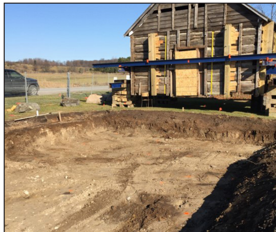
After the church was moved from its foundation and prior to being set in the new foundation. Showing excavation complete at the previous location of the church.
