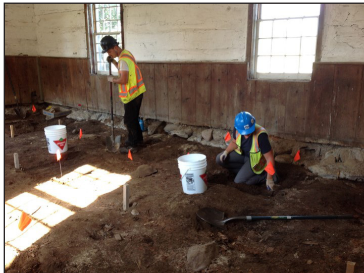
Crew members working inside the Oro AME Church before it was moved
